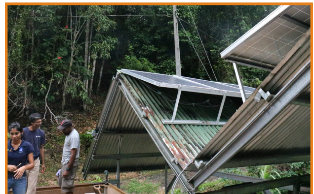
Figure 8: Solar panels on the roof of the cocoa house. 2016
